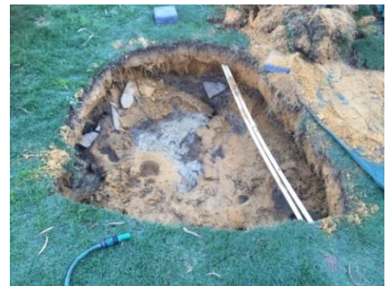
Not removing or decommissioning a septic tank
